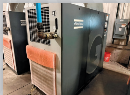
75 HP Atlas Copco GA55FF Air Compressor
