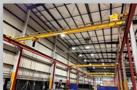
2 Ton x 37' Approx. Span x 200' Long Stewart Free-Standing Bridge Crane System
